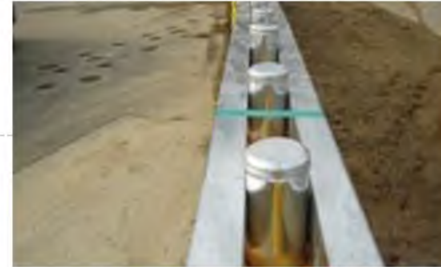
After crash of Lorry 14 ton (Not bent)
