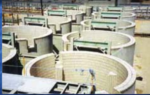
Above: Reactors lined with ceramic wear-and-tear protection
