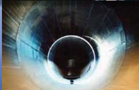
Above: Rubber-lined area of a pure gas channel
