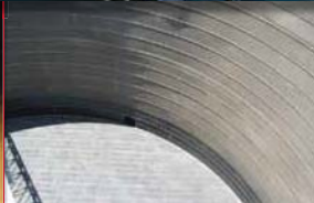
Above: Rubber-lined tank in phosphoric acid production
