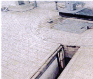
Thermoplastic channel anchored into the foundation with special details for connection them to the tiled industrial floor.
