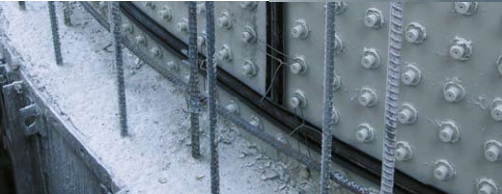
Photo on the left: The Bekaplast sheets are mounted onto the inner formwork for the concreting operation the individual sheets are still interconnected by means of special sealing strips.
