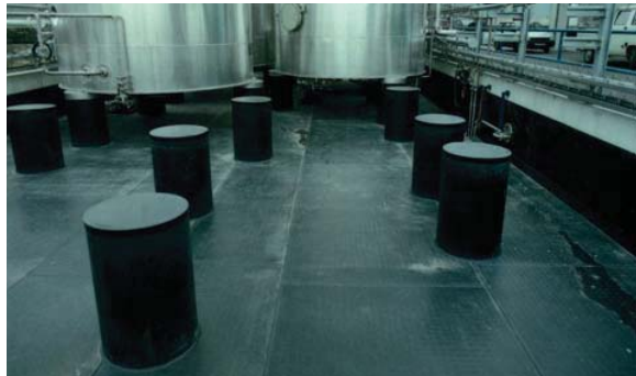
Above: BEKAPLAST™ collection tank in a manufacturing facility.
