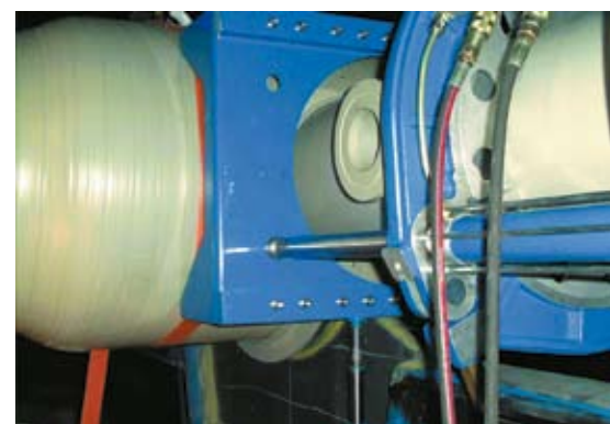
Photo below: Assembly and welding of the spray systems: In this manner a complex spray distribution system is achieved, which covers the entire area of the scrubber.
