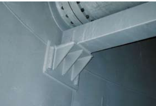
Photo above: Polypropylene supports together with the thermoplastic-lined steel girders provide support for the main ducts of the spray levels.
