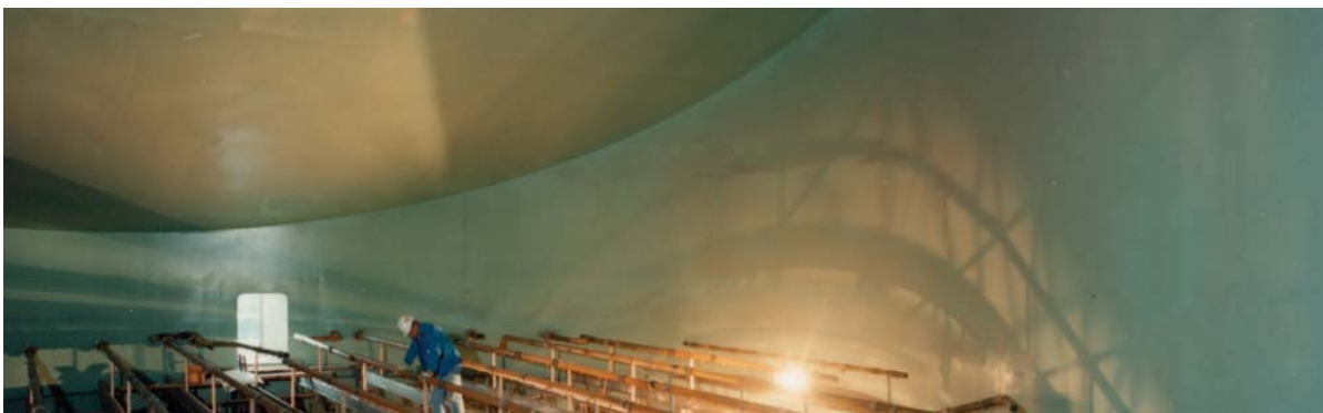
Above: Coated absorber head in a flue gas scrubber plant.
