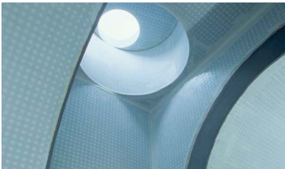
Above: Waste water collection shaft lined with natural-finish HDPE BEKAPLAST™.
