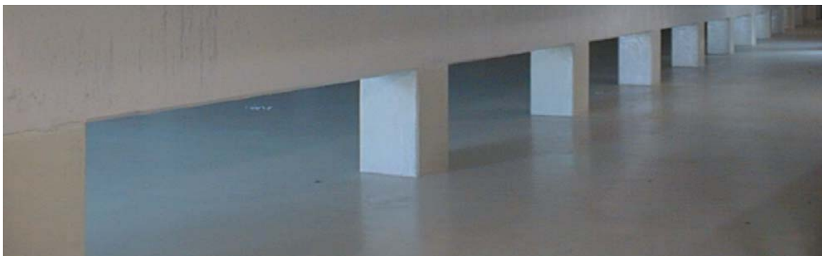
Above: Chemically and mechanically highly stressable floor coating in a zinc winning plant.
