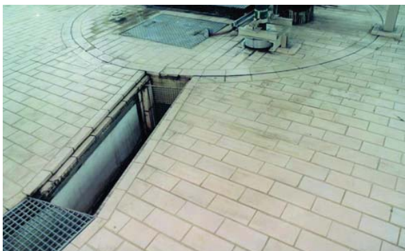
Above: Thermoplastic gutters mechanically anchored into the foundations with special detailed solutions for connection to tiled industrial floor.
