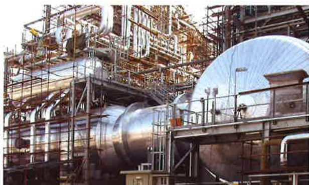
Site view of the horizontal chamber and waste heat boiler with the vertical cracking chamber
