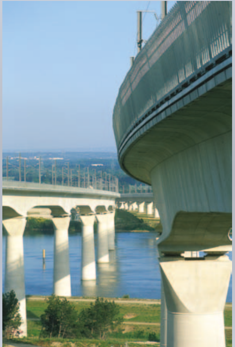
Pot bearings with vertical load monitoring system installed at the railway track of the French TGV
